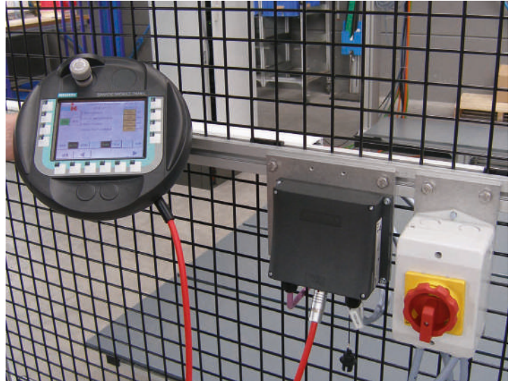
Mobile touchscreen with connection box and offset main switch
