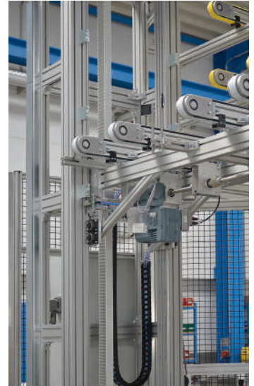
Lift for storage system
