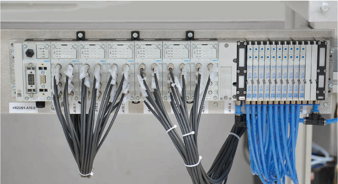
Valve terminal with input and output module
