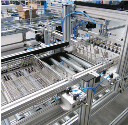
Transport in and out for a customer's measuring and packaging unit
